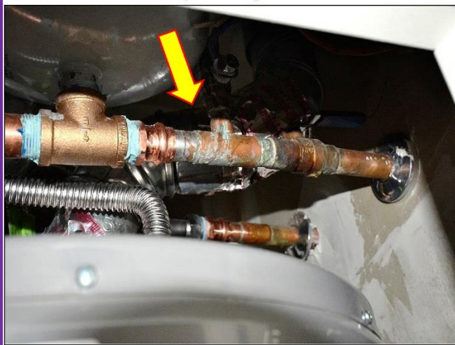
15. Valves and pipe connections above the Rheem H 2 O heater are messy with possible pin leaks and this piping should be Replaced by a Licensed Plumber.
