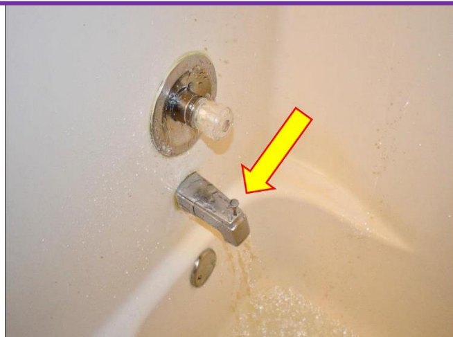
8. Bathroom Delta Bathtub/ Shower faucet is not properly working with the spout's diverter valve and it should be Replaced .
