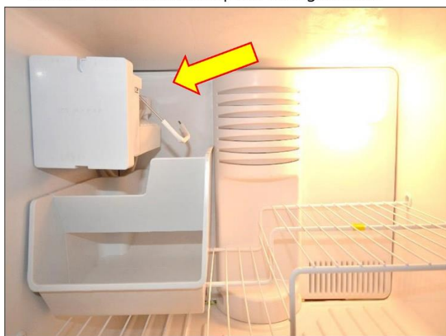
6. GE Refrigerator's Ice Maker is not properly hooked up, although there's 1/4" copper tubing found below the cabinet and above, it will need to be reestablished.
