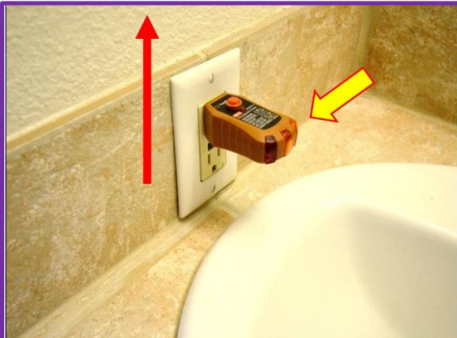
7. Bathroom GFCI receptacle is DEAD and should be relocated 6-inches above the countertop, within the drywall space as per ICC and State UEC Codes.
