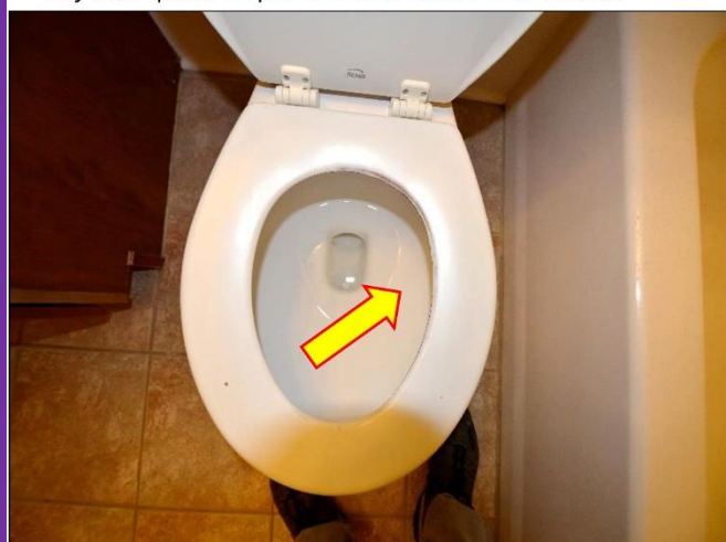
9. Bathroom Mansfield toilet seat is worn and should be Replaced .
