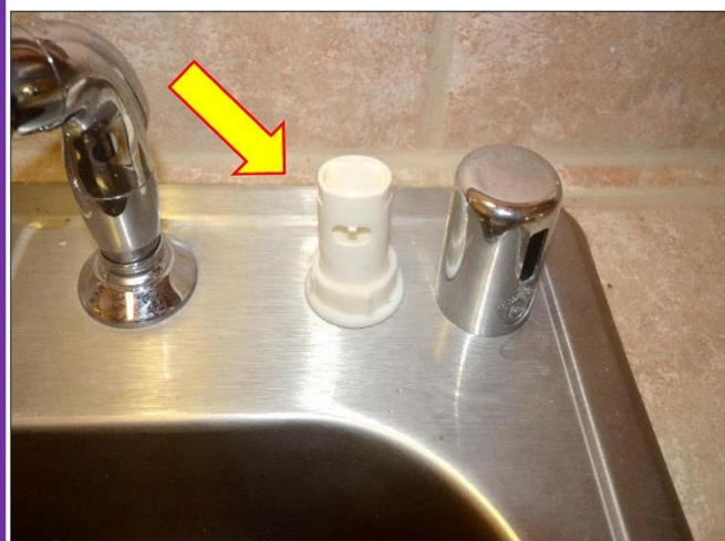
5. Kitchen sink's Air Gap is LOOSE and will need to be repaired by a Licensed Plumber.
