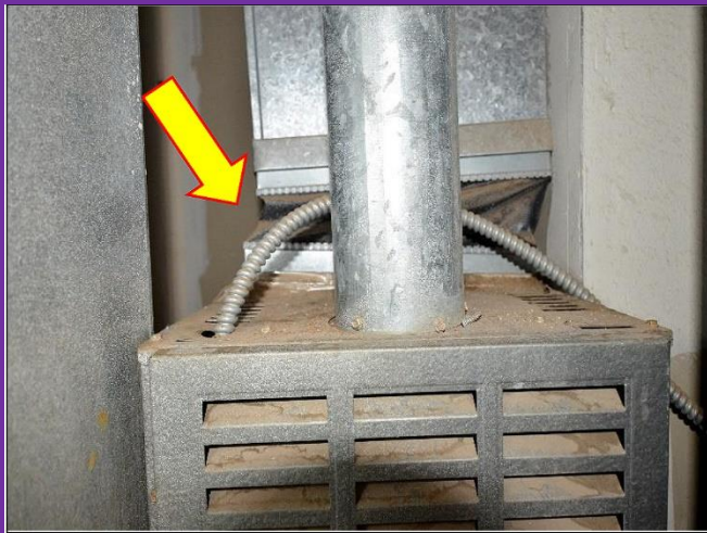
13. Plinth Jacket is LOOSE over the Carrier Furnace and will need to be immediately reset to prevent Carbon Monoxide poisoning.
