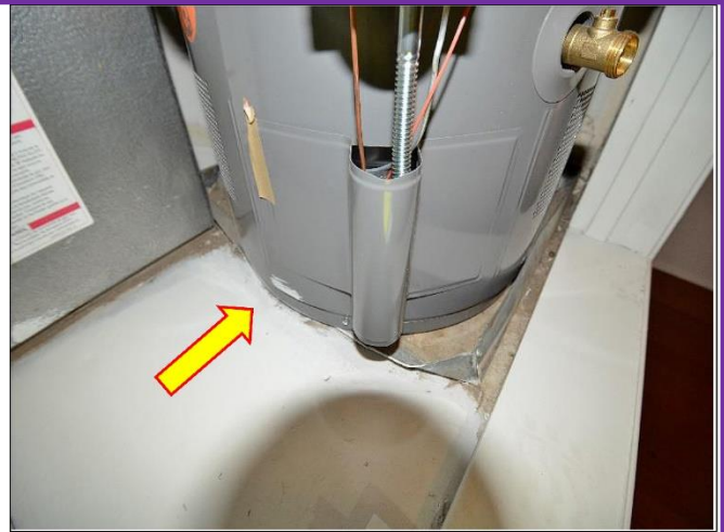
14. Rheem H 2 O heater's safety pan is crushed and will need to be Replaced and drained to an outside or waste pipe source.
