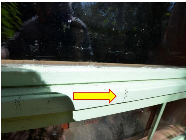
11. Some of the molding on the wood windows are showing finger joint dislodging and will need to be replaced and repainted.
