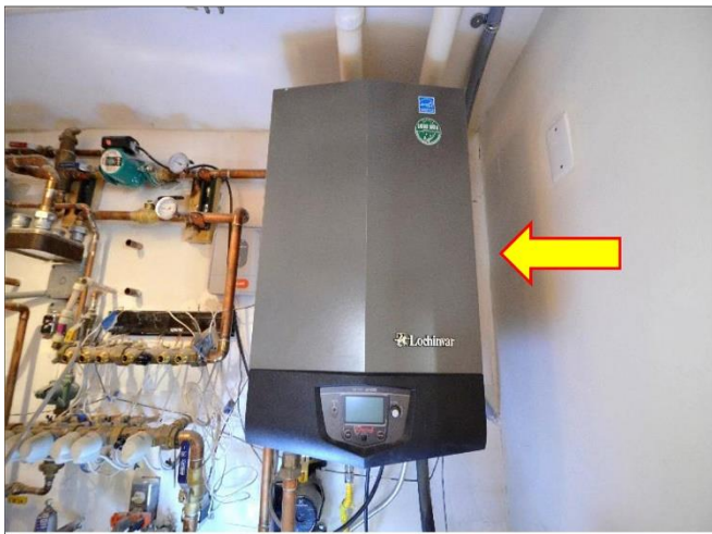
21. Lochinvar Instant H 2 O heater for radiant heating was not working at the Inspection and will need to be operational before closing this Inspection.
