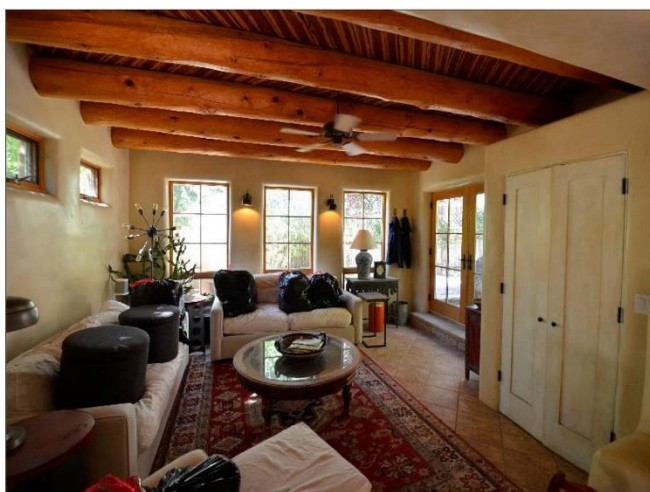
17. Living room with Vigas, herringbone latias and tile floors are in Satisfactory Condition.
