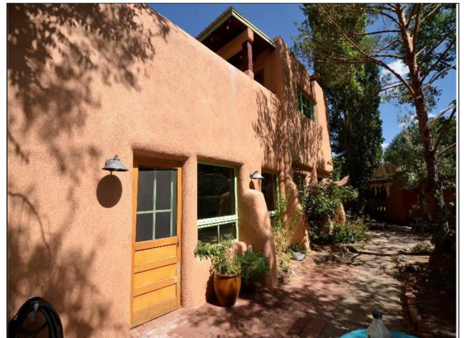
28. Front door Entry with flagstone patio pavers and stucco buttress walls are in Satisfactory Condition.
