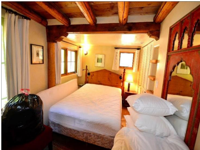
27. Downstairs Bedroom with Vigas, beam & corbels and polished concrete floors are in Satisfactory Condition.
