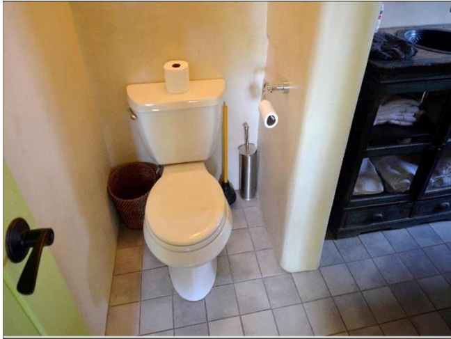
25. Downstairs bathroom with ceramic tile floors, Kohler toilet are in Satisfactory Condition.
