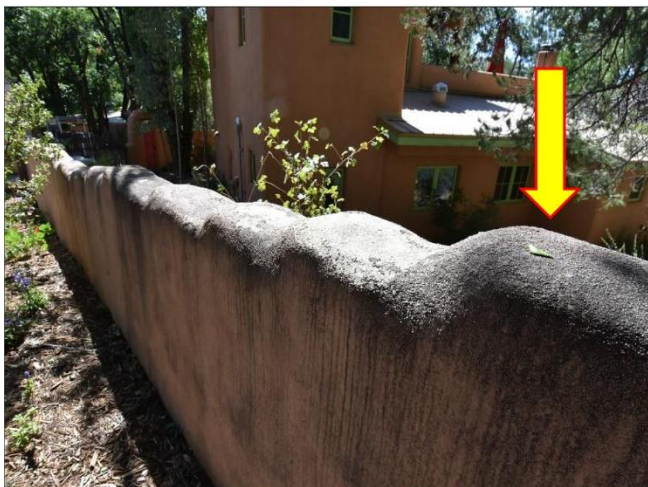
29. Garden Stucco walls are badly stained and will need to be resurfaced in time.
