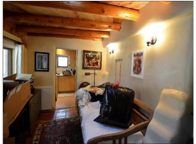
20. Office/ Utility area with Vigas and herringbone wood boards are in Satisfactory Condition.
