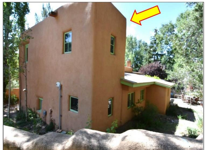
30. Two story portion of Adobe house, but the Master Bathroom is made of frame walls.
