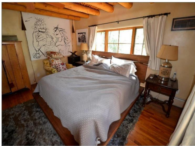
15. Master Suite Bedroom with wood floors, Vigas and decking is in Satisfactory Condition.
