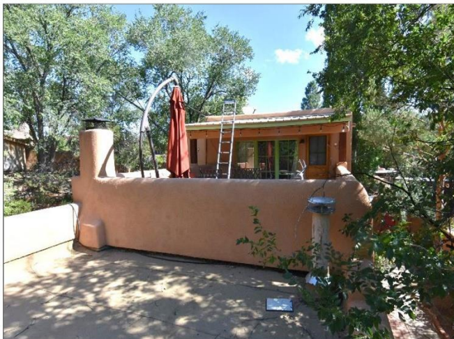
5. Lower Torch-down roof over Living and Dining rooms is in Satisfactory Condition.
