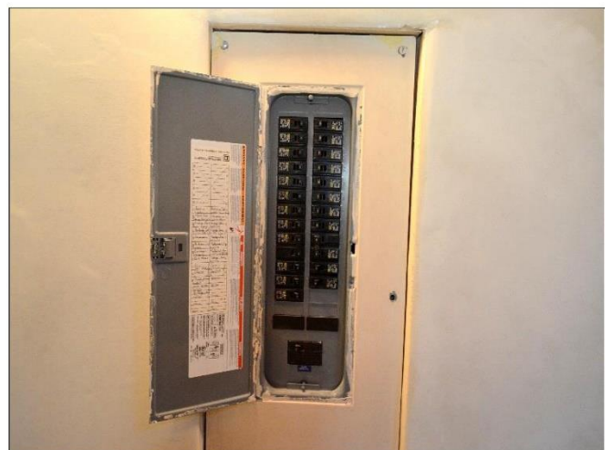
24. 100Amp Panel is safe and properly wired for the House.
