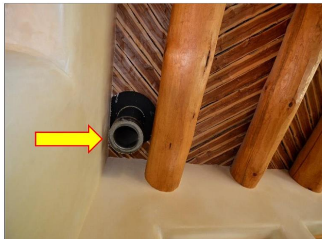
12. Wood burning metal flue should be covered underneath.
