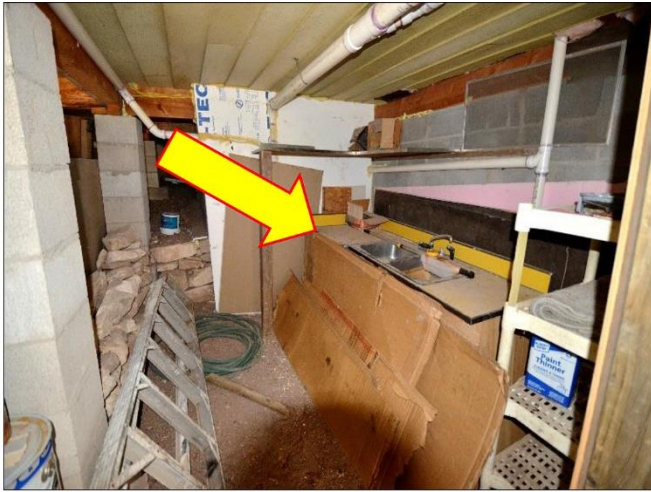
13. Crawl Space showing a discarded sink & counter that should be removed.
