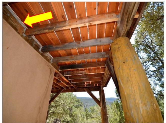
18. Under deck at the ground level with Viga Posts that should be refinished as well. Ledger is lag screwed to the wall and is apparently safe.
