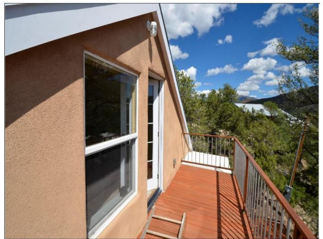
16. 3rd Floor decking that is also dry and will need an oil seal with Behr Products to prevent weathering at least every 3-years
