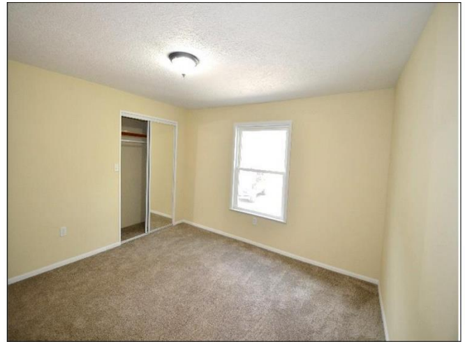
32. 2nd Floor Master Bedroom with carpeting and CertainTeed Vinyl windows are in Satisfactory Condition.
