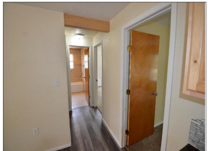
36. 2 nd Floor Hallway between Kitchen and Master Suite is in Satisfactory Condition.
