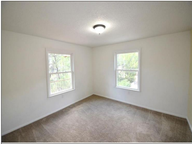
31. 2nd Floor Bedroom with carpeting and CertainTeed Vinyl windows are in Satisfactory Condition.
