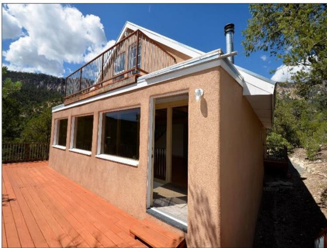
15. 2nd Floor decking that is dry and will need an oil seal with Behr Products to prevent weathering at least every 3-years
