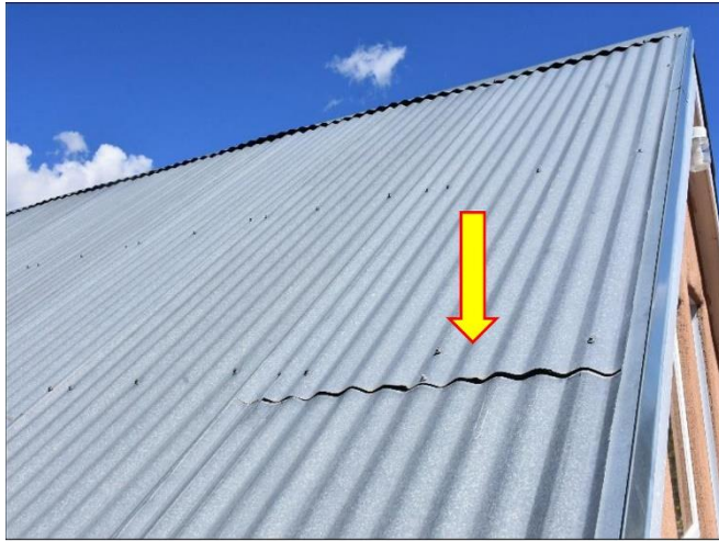
1. Corrugated zinc panel roof was installed with recycled materials and may need immediate attention to prevent leaks.
