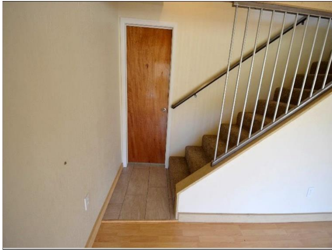
25. Staircase to the 3rd floor have a 3-way switching as per code and is in Satisfactory Condition .
