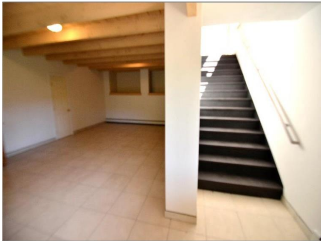
27. Main 4-foot Staircase from Basement to 2nd Floor with a single handrail and 3-way switching as per code is in Satisfactory Condition .
