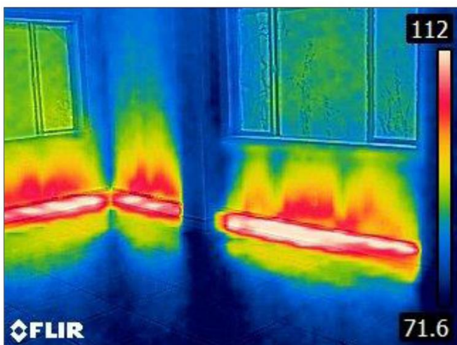
53. InfraRED Thermal Imaging of the Radiant Baseboard Heating on the 1st Floor, (Basement Room).
