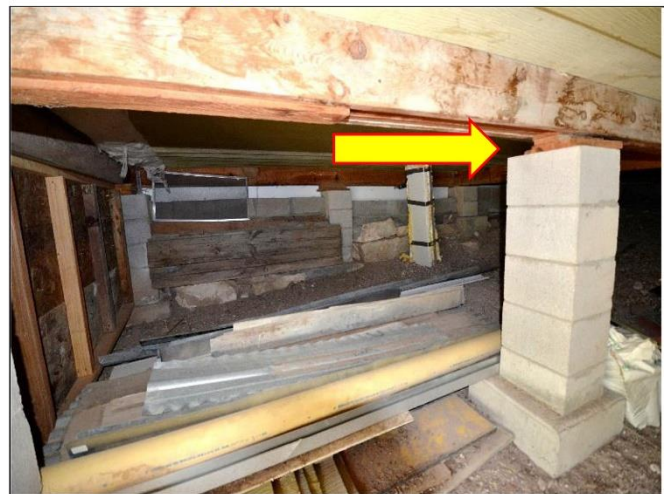
6. CMU Block piers throughout the Crawl Space should have steel strong ties engineered for better seismic supports. Shims were loose.
