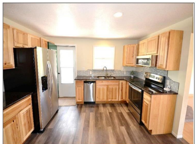
24. Kitchen, all electric with quality cabinets and vinyl flooring are in Satisfactory Condition . Split Floor level from the Kitchen to Living can be problematic.
