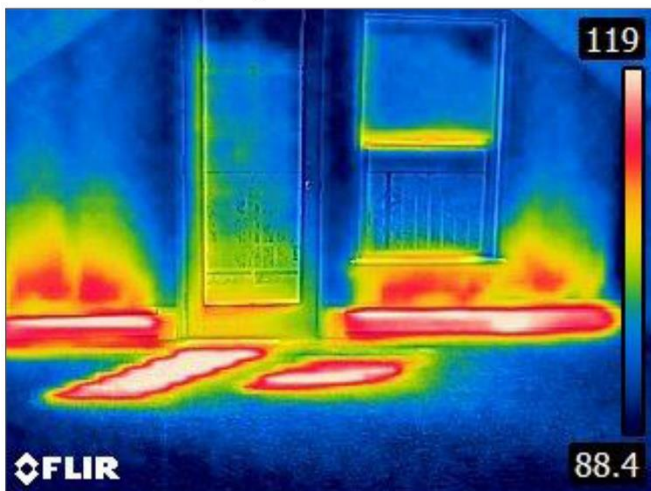
51. InfraRED Thermal Imaging of the Radiant Baseboard Heating on the 3rd Floor, (Bedroom).
