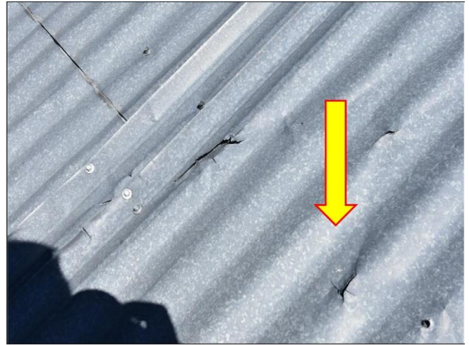
2. Corrugated zinc panel roof was installed with recycled materials showing tear and small holes will need immediate repairs.
