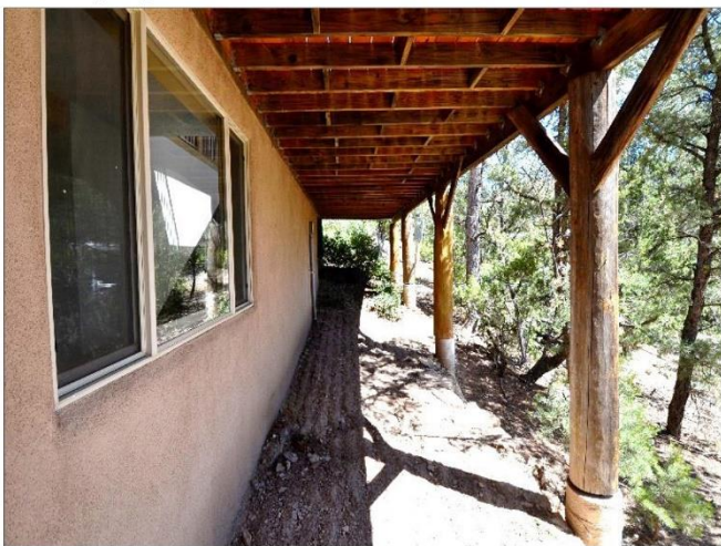
17. Under deck at the ground level with Viga Posts that should have high strength grout packed under the posts to prevent rust to the 1/2" bolts.
