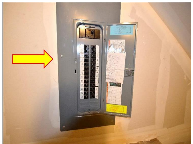
30. Electric 200Amp Panel found under the Main Staircase on the Basement level is in Satisfactory Condition .
