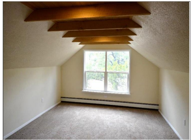
34. 3rd Floor Bedroom with cathedral beam ceiling, carpeting and CertainTeed Vinyl windows are in Satisfactory Condition.
