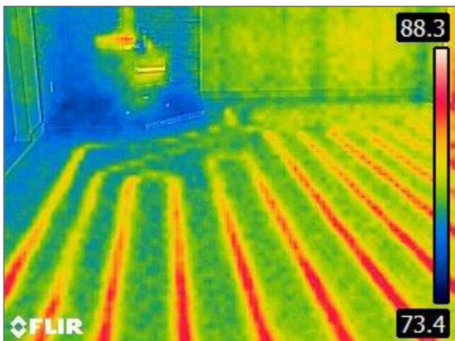
45. InfraRED Thermal Imaging of the Radiant Heating the 2 nd Floor, (Main Floor) set with Warmboard set under Pergo flooring.
