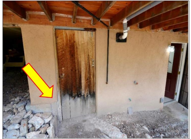
8. Separate door to the Mechanical Area under the House will need an oil seal to prevent weathering.
