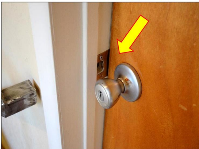
35. 3rd Floor door to Bedroom is stuck and does not close.
