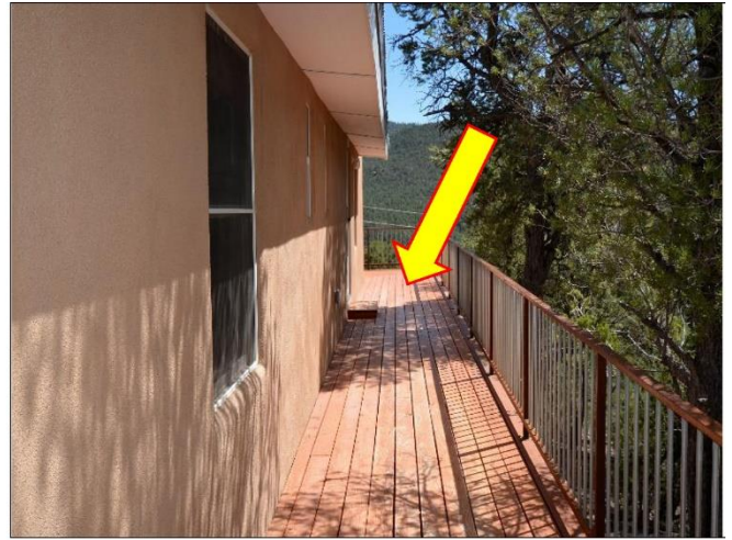
14. 2nd Floor decking that is dry and will need an oil seal with Behr Products to prevent weathering at least every 3-years.
