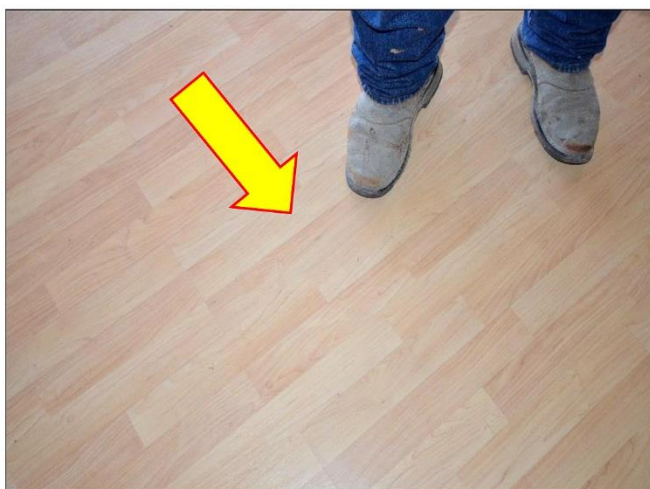
23. Some areas of the Pergo flooring that are slightly spongy and it's recommended in the future to exchange the flooring material with a better surface.
