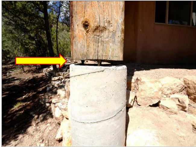
19. Example of Viga Posts that should have high strength grout packed under all of the posts to the concrete piers to prevent rusting to the 1/2" bolts
