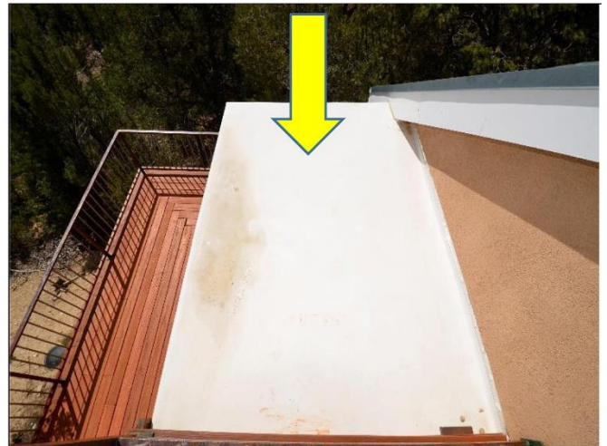
4. TPO roof membranes were installed at both ends of the upper deck roof and are in Satisfactory Condition .
