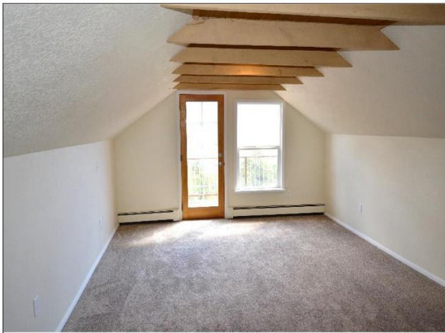
33. 3rd Floor Balcony/ Office with cathedral beam ceiling, carpeting and CertainTeed Vinyl window and glass door to deck are in Satisfactory Condition
