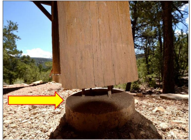
20. Example of Viga Posts that should have high strength grout packed under all the posts to the concrete piers to prevent rusting to the 1/2" bolts.
