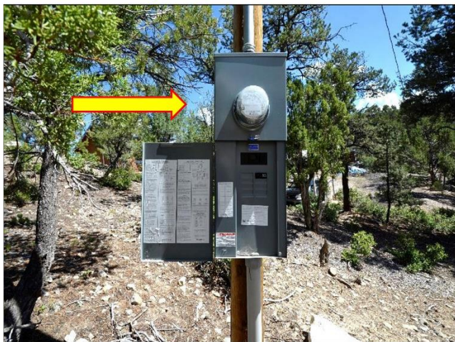
29. Utility PNM Service Meter with Main 200Amp Discount is in Satisfactory Condition .
