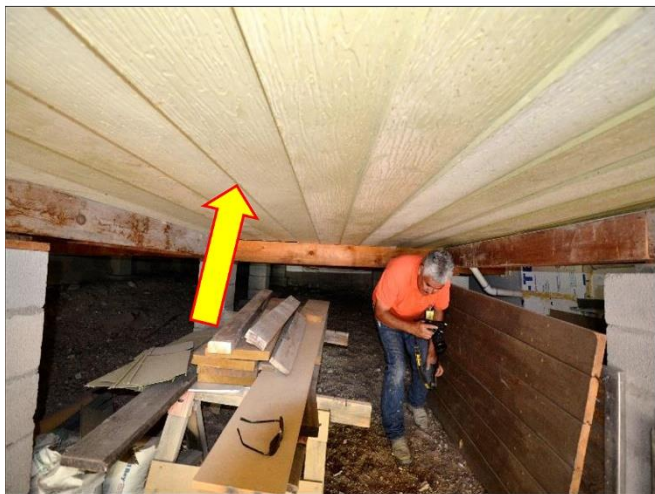
5. Ceiling coverings by using recycled aluminum siding to cover the rafters conceals assumed insulation but cannot be verified.
