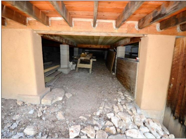
7. Opening to the Crawl Space that should have doors installed for security purposes to keep animals from damaging the space within this rural environment.
