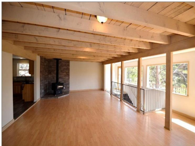
21. 2nd Floor Living Room with beams and T&G decking and Pergo flooring.
